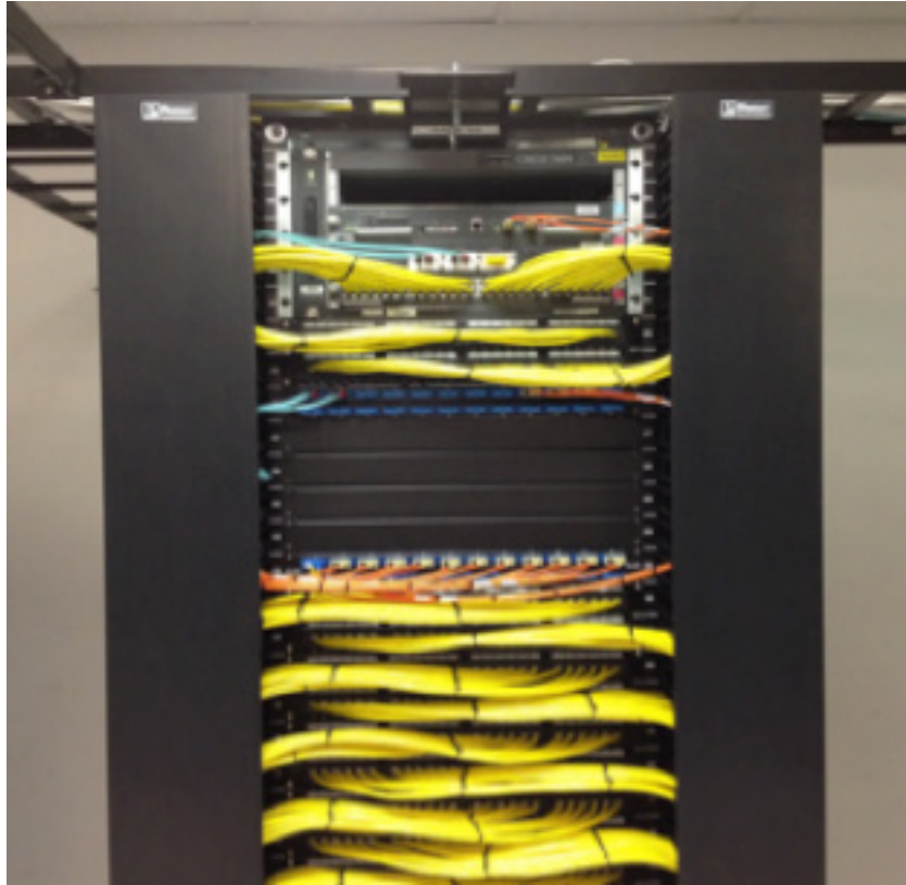
Network Cabling in Dallas, TX Synthesis Data Backup Facility
